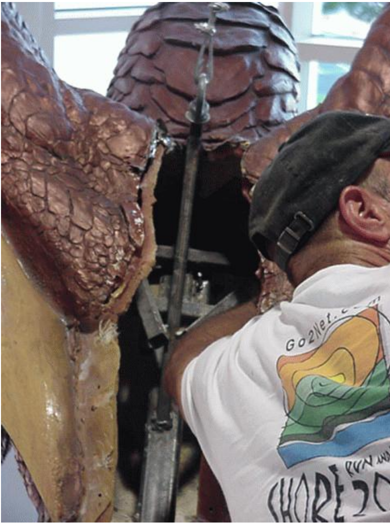
Hooking up cables to the Dragon's spine.
